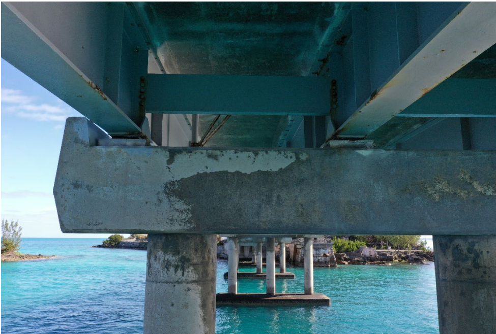
Photograph 12 – Bearings 15 and 16 showing cracking of the concrete plinths
