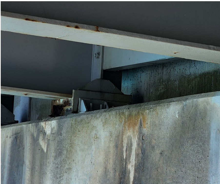
Photograph 20 – Bearing B31 showing corrosion of steel plate girder above.
