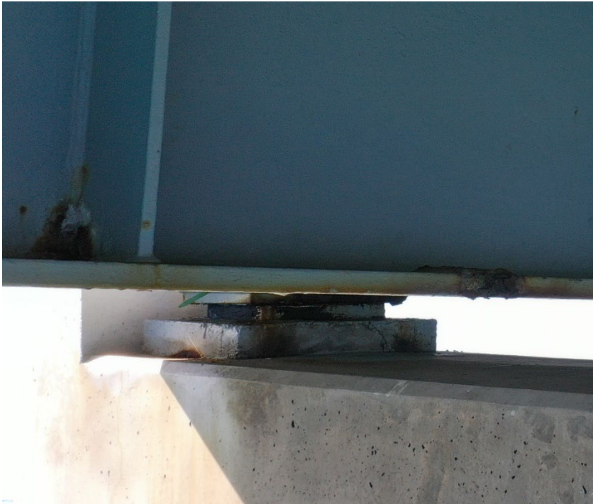
Photograph 7 – Bearing B9 showing vertical and diagonal cracking.
