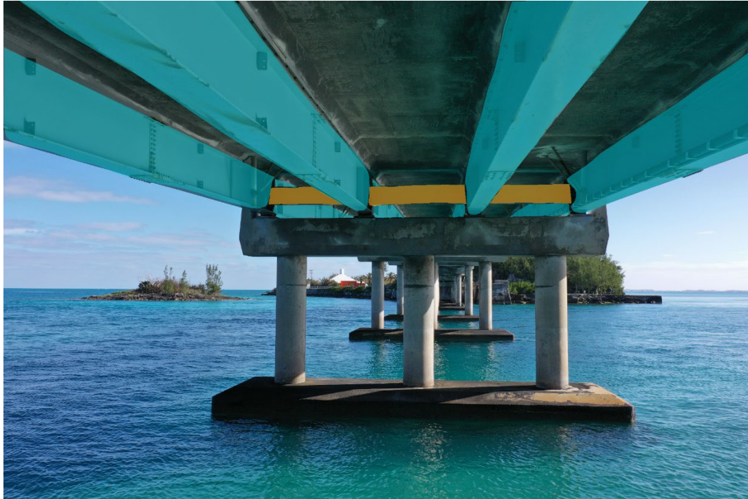
Figure 2. View of Watford Bridge Soffit. Showing Beams to Be Recoated In Each Span.
