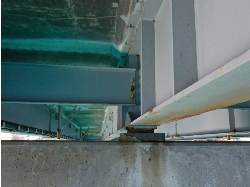
Photograph 8 – Bearing B10 showing a diagonal crack.
