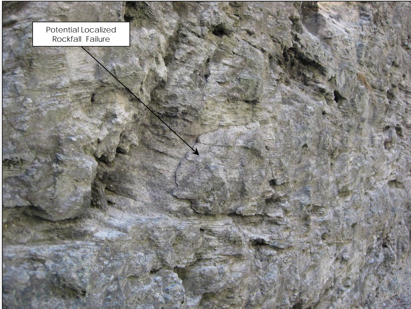
FIGURE 6 PHOTO SHOWING PARTIALLY DETACHED AND LOOSE ROCK BLOCK
