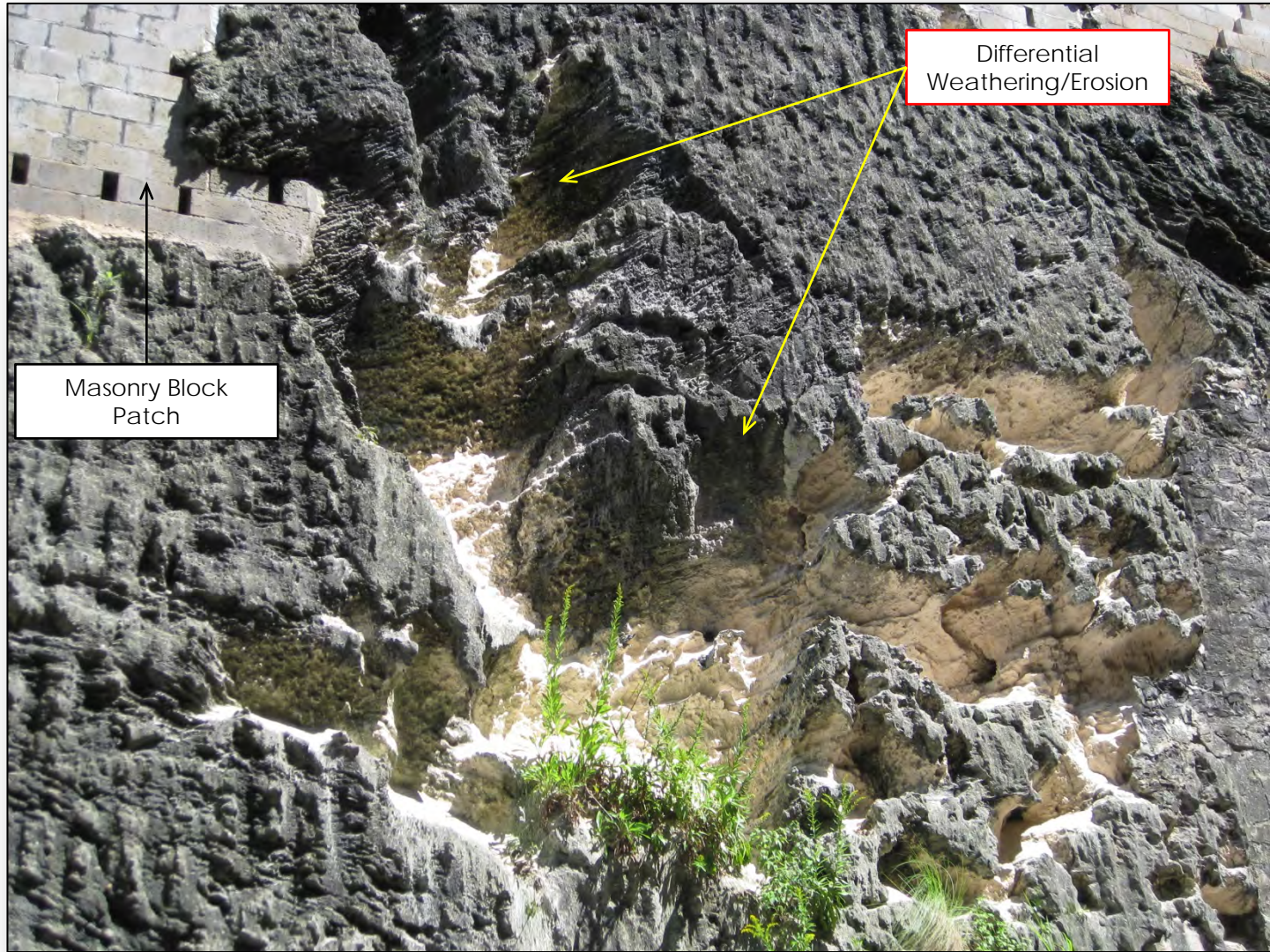
FIGURE 3 PHOTO SHOWING DIFFERENTIAL EROSION AND MASONRY BLOCK PATCH
