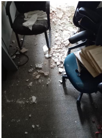
BGL- 33: Room 105, Ceiling Damage
